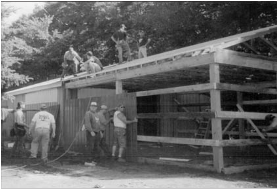
Volunteer workers place siding on the addition to the Leach family barn. (Photograph courtesy of Debbie Swaffield)
