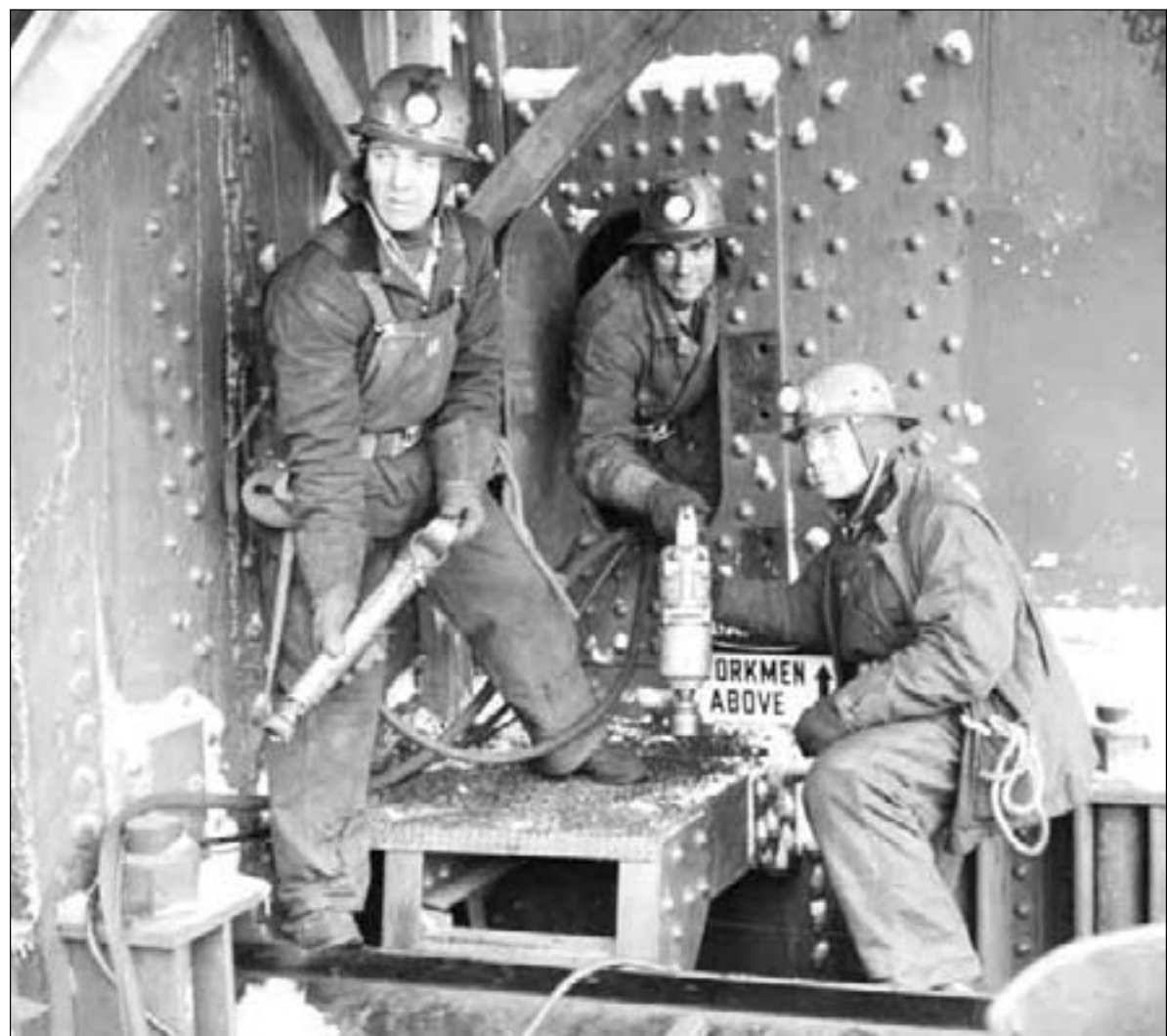
As snow dusts a tower during construction of the Mackinac Bridge, three unidentified riveters work to place the six million rivets that permanently connect the tower. (Photographs courtesy of the Mackinac Bridge Authority.)
