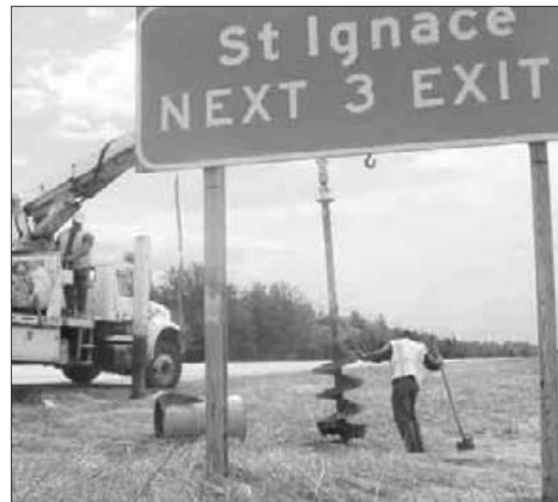
Holes are being drilled for new signs that will replace current ones along both the northbound and southbound lanes on I-75 between Sault Ste. Marie and St. Ignace. Action Traffic Maintenance of Flint is conducting the work, with employees Foreman Don Campbell (left) of Almont and Lyman Krump of Chesaning.
