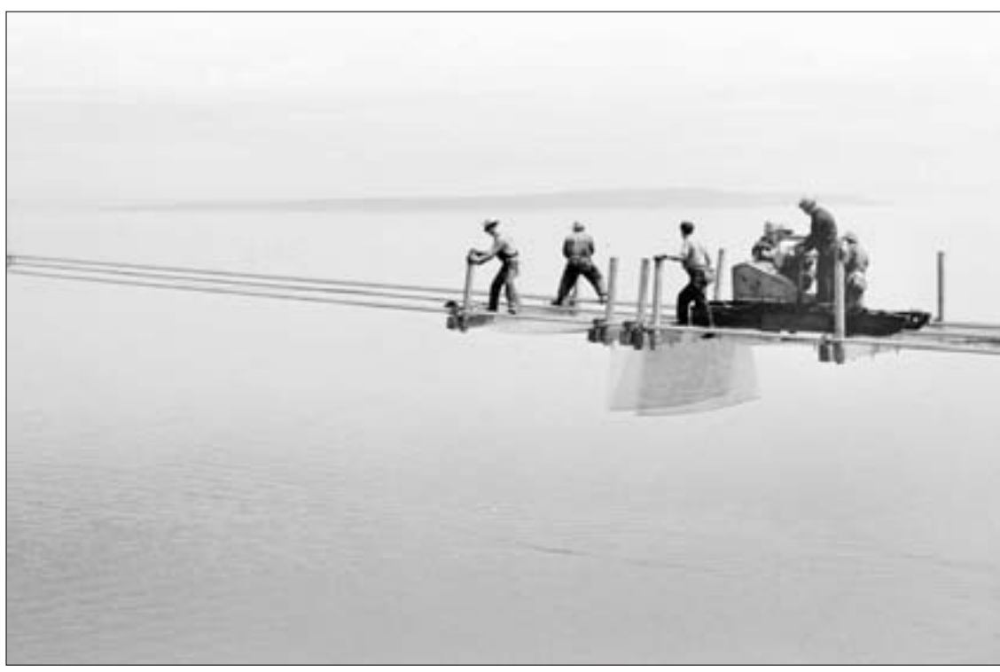
From 550 feet above the Straits of Mackinac, ironworkers built a catwalk that swooped down to approximately 200 feet above the water. With Mackinac Island in the background, ironworkers focus on building the catwalk, which was used in the construction of the two main support cables for the Mackinac Bridge. Since the cables weighed 12,500 tons and could not be lifted into place, they were assembled on-site. Each cable consisted of 12,580 wires and each wire was approximately the diameter of a pencil. (Photograph courtesy of Mackinac Bridge Authority)
