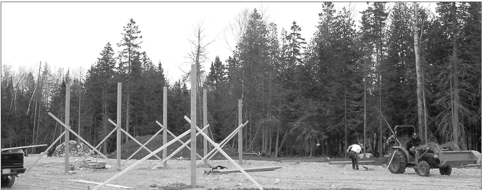
Todd Reid (on tractor) and Ken Bailey begin work on the new Clark Township Recreation Park pavilion in Cedarville Monday, April 30. They raised the frame for the 30-foot by 40-foot, open-sided building behind Clark Township Hall, to the west. The pavilion was donated by McMaken Carpentry of Cedarville, and is the first facility to be built in the new park. Ball diamonds and a well are expected to follow this summer.
