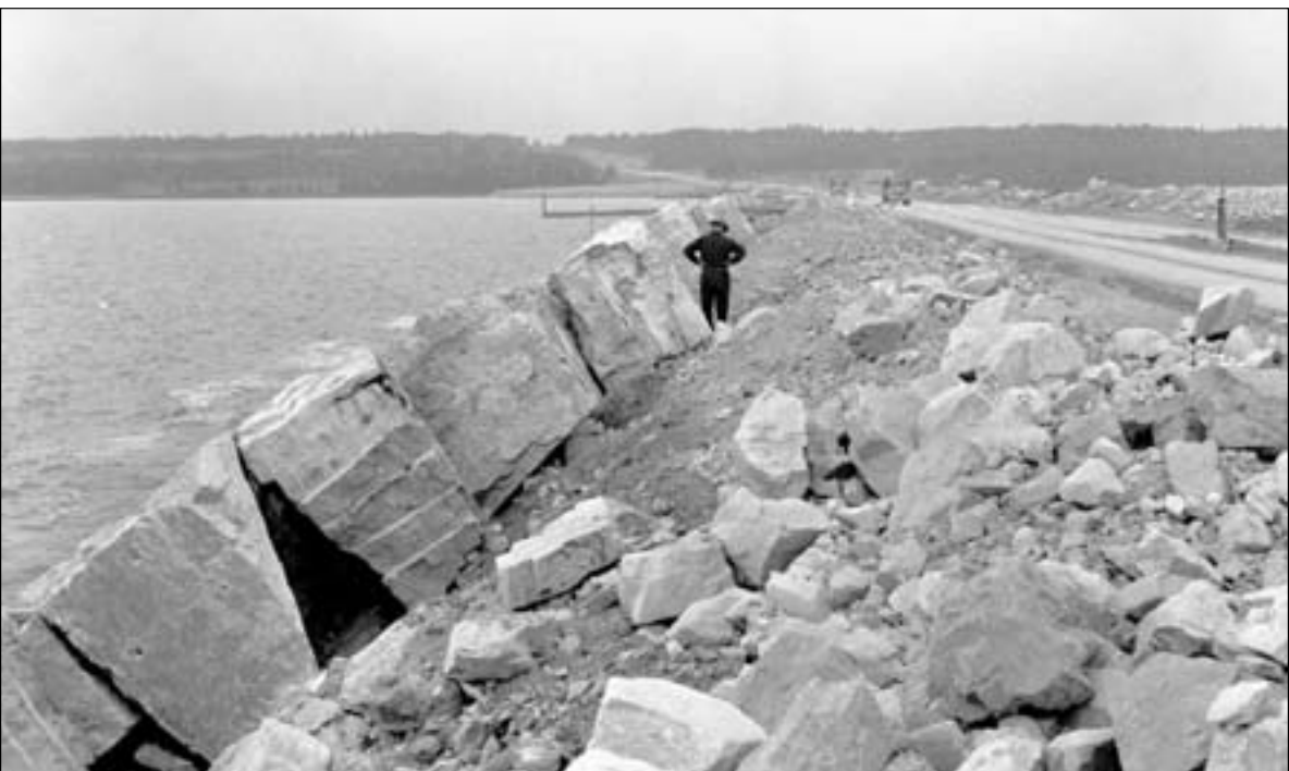
With WWII suddenly underway, construction on the causeway/ferry dock extending south from the Upper Peninsula shoreline ended for lack of trucks to haul materials. Large rocks were deposited along the banks to keep winter weather from washing the construction away, and the quarry that supplied them had trouble keeping up. But the war also diverted materials needed to complete the ferry slips at the end of the causeway, so wood was substituted for steel. Meanwhile, the ferries continued to land at Dock 2 in St. Ignace. (Michigan Department of Transportation)
