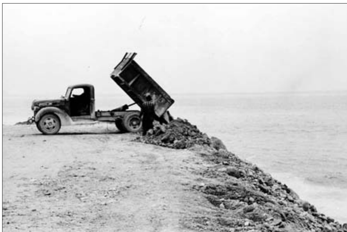
To catch up with causeway construction, Johnson and Greene worked two shifts hauling rock to the site just south of St. Ignace. The causeway would reach its maximum length during this period, before the war brought construction to a standstill. (Michigan Department of Transportation)
