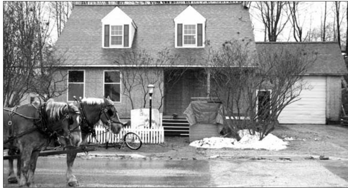
In preparation for new siding, plywood covers Mackinac Island's old medical center on Market Street. The building is being converted to housing for Island police. The fiber cement siding planned for the historic district structure raised concerns of city planners Tuesday, January 8.
