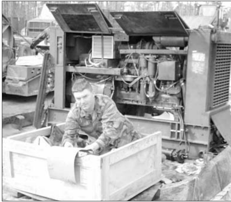
Construction Mechanic Second Class (CM2) Thomas Wilk replaces a blown oil pan gasket on a generator at Camp Shelby, Mississippi. Enrolled in active duty with the Navy, CM2 Wilk is assigned to Alfa Company, Naval Mobile Construction Battalion (NMCB) 133, based in Gulfport, Mississippi. Construction mechanics are responsible for field repairs on large equipment. CM2 Wilk will deploy this summer with the USNS Mercy, a hospital ship, conducting humanitarian missions in the Pacific Theater. Seabees from NMCB 133 will be assigned to perform humanitarian construction on shore. He is the son of Mary Wilk and Randy Stempki of St. Ignace. (Photograph by Lt. Steven Voris)
