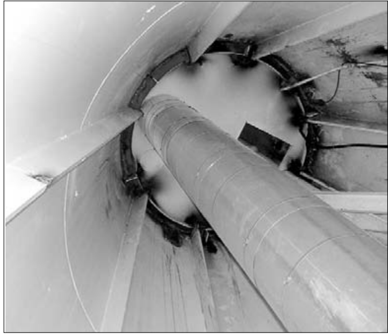
When the Evergreen Shores water tower was raised 26 feet in 2007, Pittsburgh Tank and Tower veered from the engineering design, Bill Dixon, president of Dixon Engineering Inc. of Lake Odessa told St. Ignace City Council Monday, June 16. The on-site modifications, he said, affected the structural integrity of the tower. Internal stiffeners shown in this picture, taken March 12, 2007, should have been placed at equal distances, but were not. The tower cracked during a windstorm March 1, 2007.
