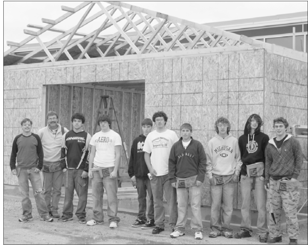
One of three LaSalle High School construction classes are building this garage for storage behind the school. The first-hour class includes (from left) Nick Gould, teacher Lynwood Leightner, Rob Grondin, Bob LaDuke, Robert Sayles, Frank Beaudoin, Jeff Gamble, Justin Frazier, Ryan Waldrup, and Jake Gawne.
