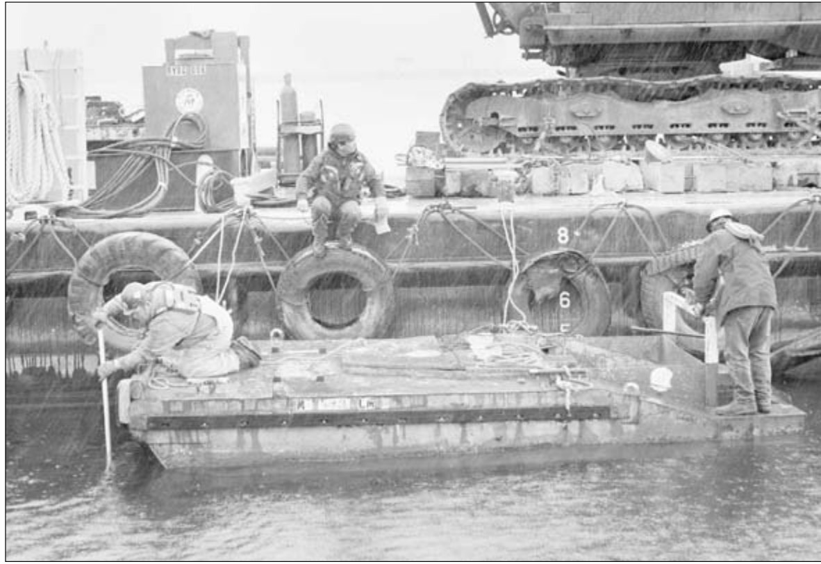
From a small working barge, Ryba Marine crew members work in pouring rain to begin the process of replacing a pylon at the Mackinac Island marina.
