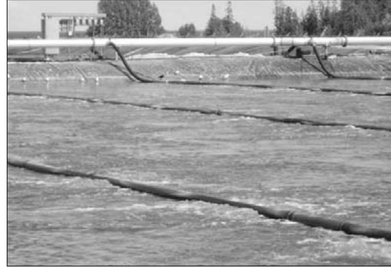
An aerator system circulates air through one of the lagoons at the St. Ignace sewer plant, adjacent to the Mackinac County Airport. Some of the plant's ponds, like this one, were cleaned out of sludge build-up and the liners were replaced during a recent round of improvements.
