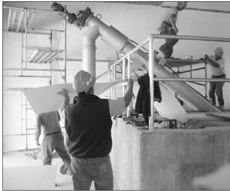
Workers from DeVere Construction Company put finishing touches last week on the new building at the sewer plant, which will house the new screening and ultraviolet disinfectant systems to clean wastewater in St. Ignace.
