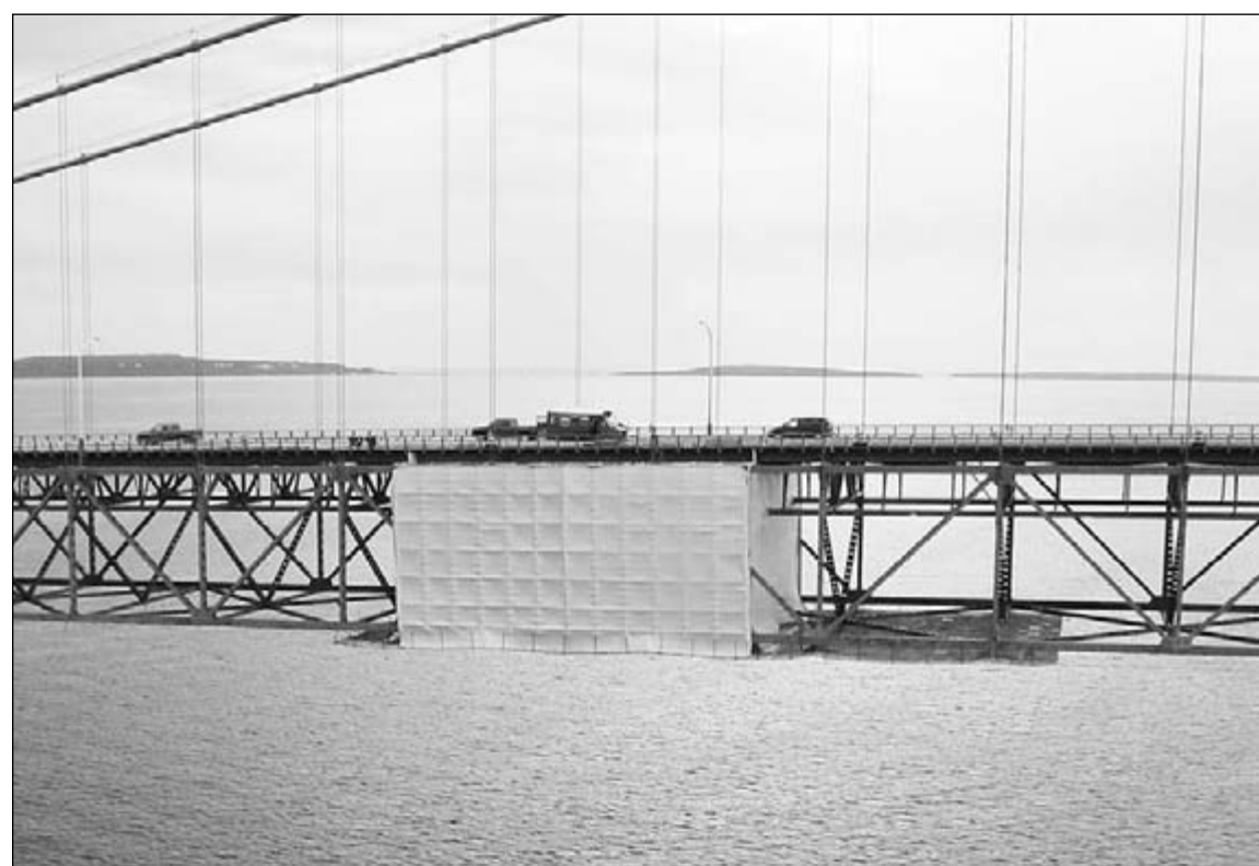
A containment system surrounds the area where sandblasters and painters work on the Mackinac Bridge. The Safe-Span work platform and scaffolding combination, which allows access for workers and catches any debris before it falls into the water, is a first for Mackinac Bridge painters. (Abhe & Svoboda, Inc. photograph)
