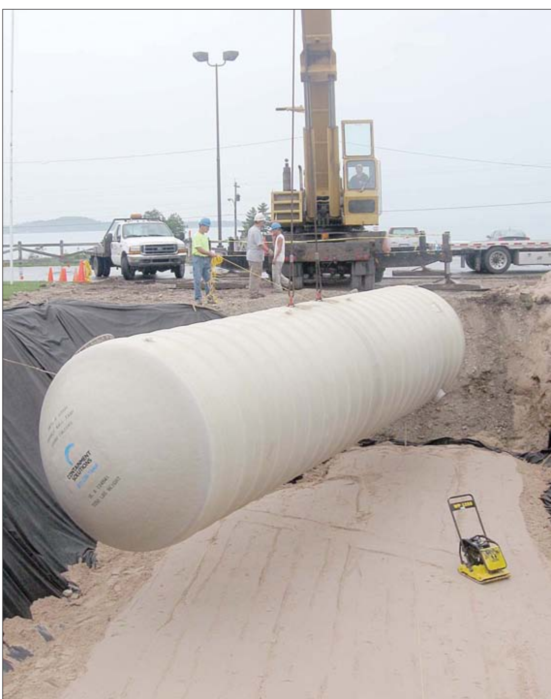
Workers from U.P. Environmental Services and crane operators from Vandermissen and Son, from Bark River and Escanaba, lower a 12,000-gallon double-lined fiberglass fuel tank into a waiting hole next to the Mackinac County Airport terminal. The airport is getting two new tanks, one of which will offer a new type of fuel at the airport -- jet fuel.
