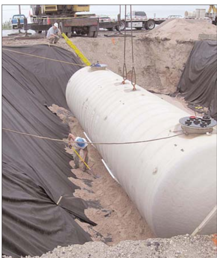
Workers from U.P. Environmental Services work to secure the position of the jet fuel tank placed in the ground next to the Mackinac County Airport terminal Thursday, August 20. A second tank, which will hold 15,000 gallons of 100-octane gasoline, will be placed next to it, replacing the current tank, which is about 20 years old.
